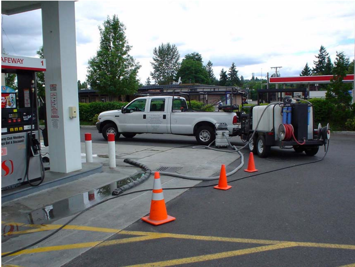
Figure 106. Pressure Wash Water Recovery System
